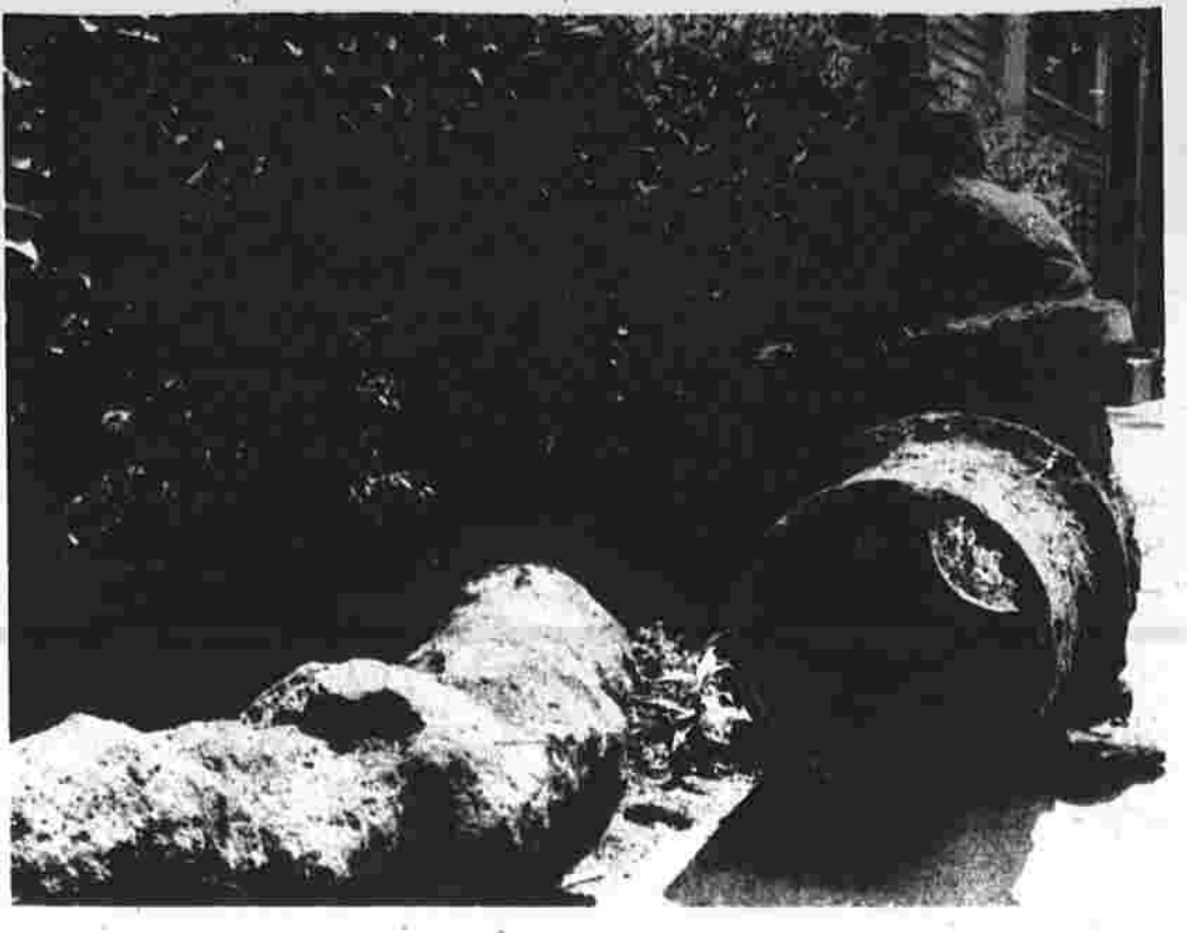
The overhaul of the town's water pipes is continuing, with the removal of the town's water pipes. This badly corroded pipe was removed near the corner of Spruce and Birch streets. (Herald photo by Hendrix)
